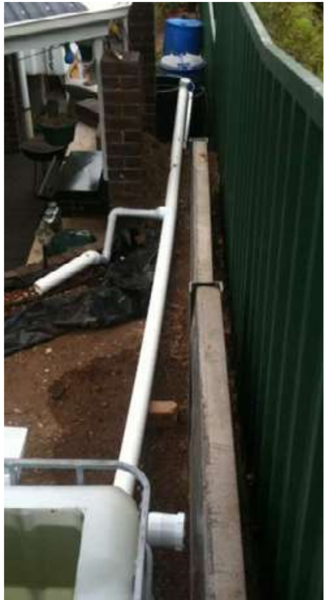
Side view showing where they are situated in the backyard. Home made level control skimmer boxes. 90 mm storm water PVC with removable ends for cleaning
