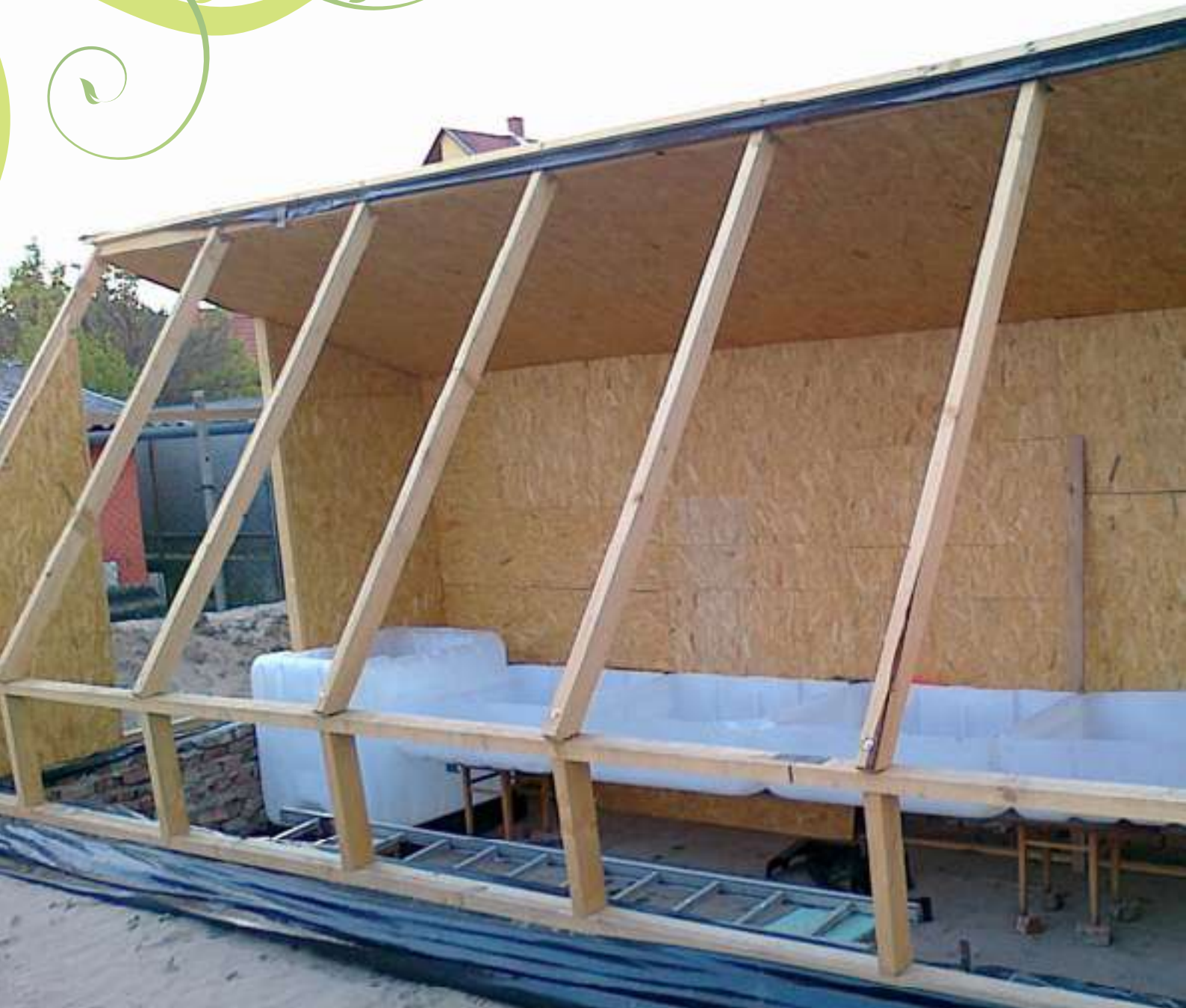
With the structure well on it's way to completion, time to check how the system is going to fit
