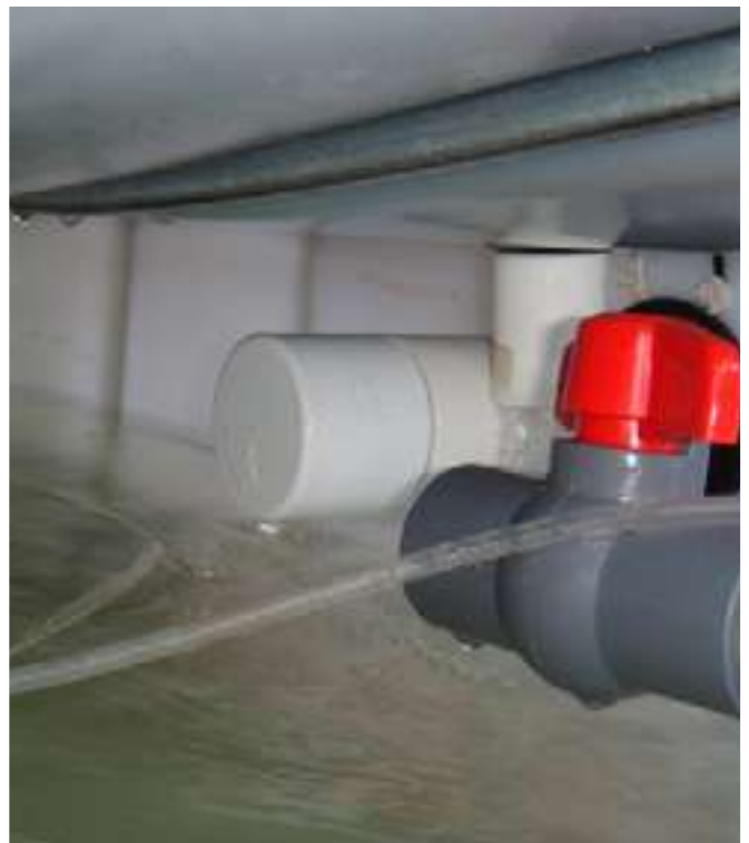
Piping and fittings under the bed
