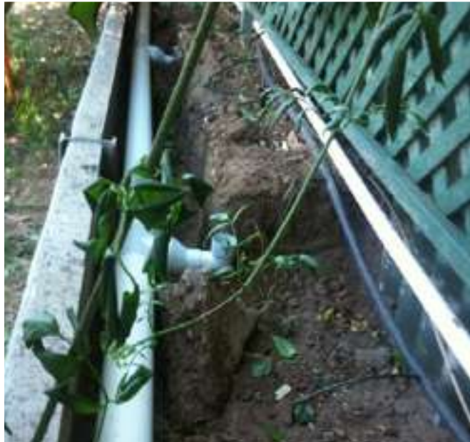
Drain from the barra grow bed ready to be hooked into the new IBC drain
