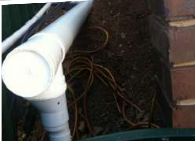
Looking from the filter and sump module
