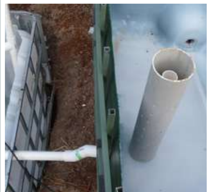
Details of the standpipe and media guard in the growbed, with the drain pipe coming out of the bottom into the sump
