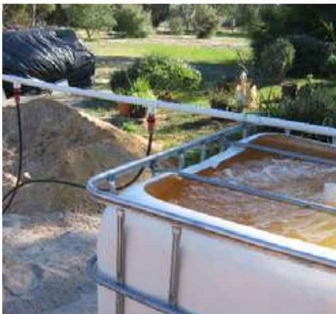
Tank and polypipe returns
