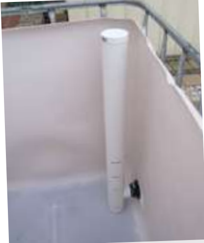
Super long standpipe and standpipe surround
