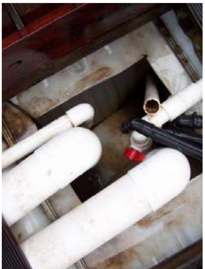
Pipework is hidden discretely under the decking and out of sight
