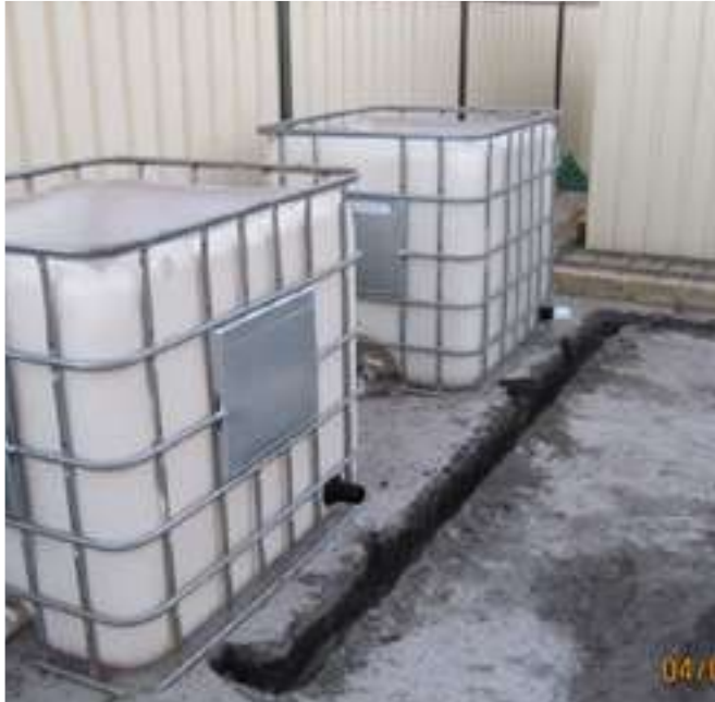
1st 2 IBC's in place with tank fittings installed and trenches dug ready for pipe work
