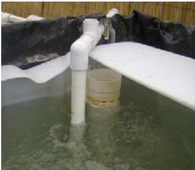
Here we can see the bubbles from the venturi sucking air into the water stream. Also the 90mm Solids lift overflow in the background
