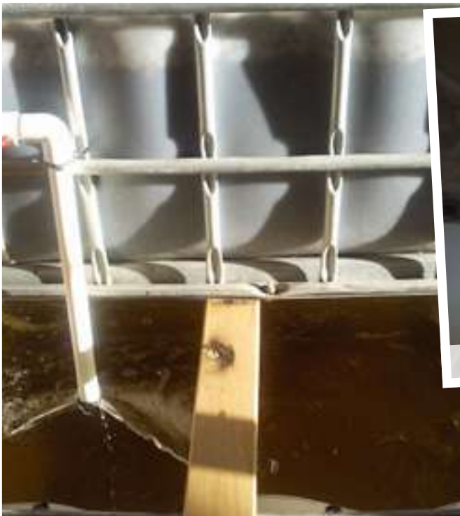
Timber supports must be heavy duty to support the weight of heavy media beds
