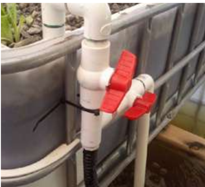
Water flows to the growbed and tee returns water to the fish tank
