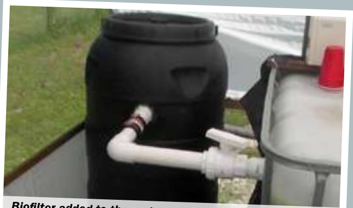
Biofilter added to the system once it was up and running
